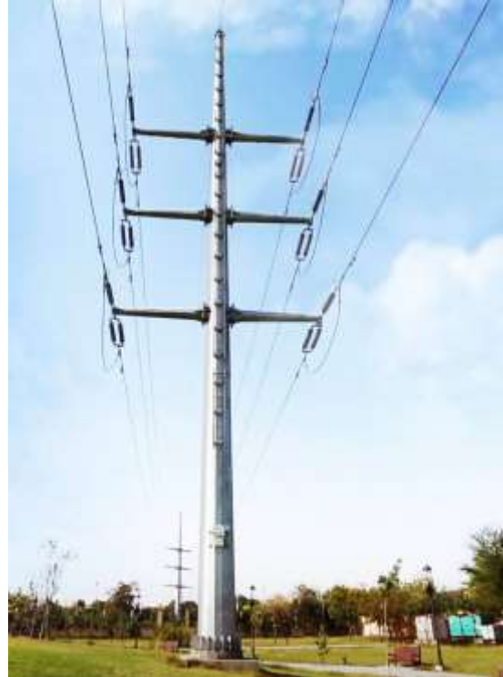
Tubular pole (monopole) tower
